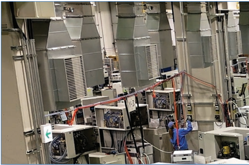
Environmental Air Management System
